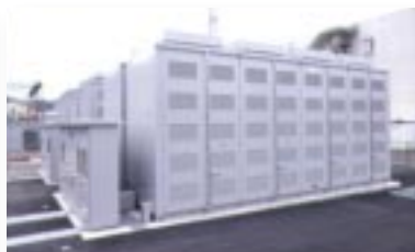
Lower-cost 6 MW-class NAS battery system (TEPCO's Ohito substation) This prototype displays a 20% improvement in energy density over previous versions.
