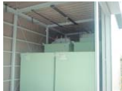
Storage facility for equipment using PCBs (Chita Plant)
