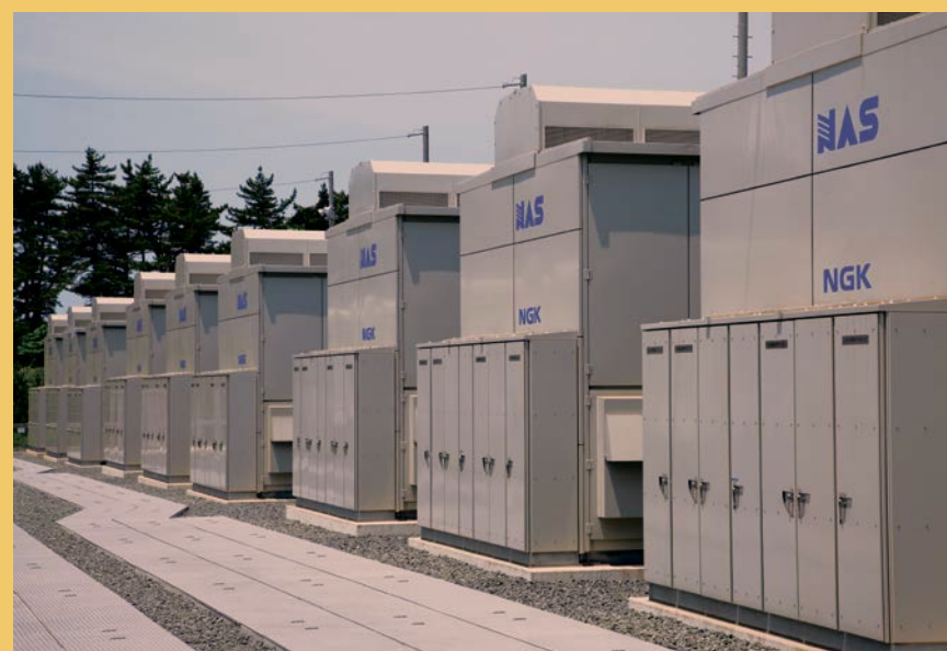
The compact NAS battery is one of the most mature and reliable technologies for grid-scale battery storage.
